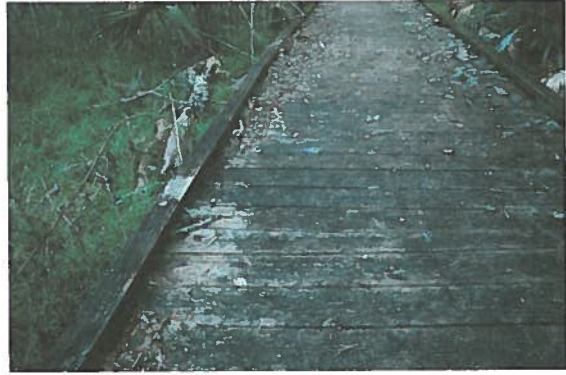
Deterioration of treated pine boardwalk
