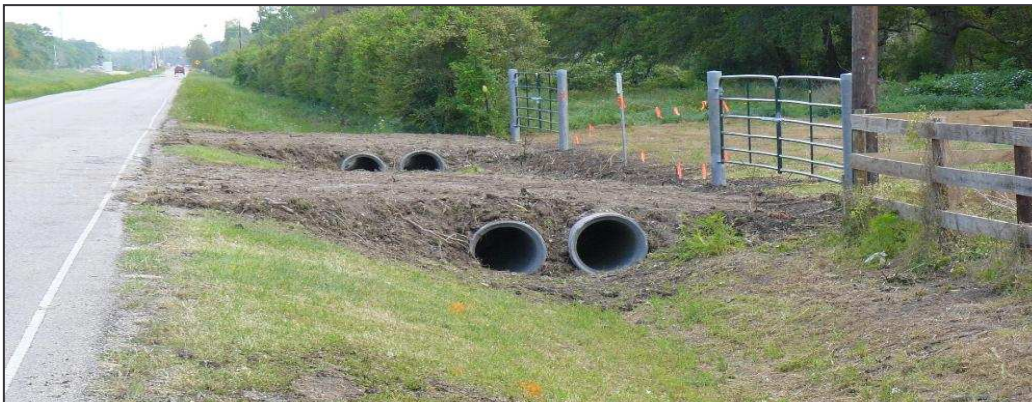
Dow Woods Unit parking lot extension under, under construction, looking south. Note the wide gates designed to accommodate school busses.
